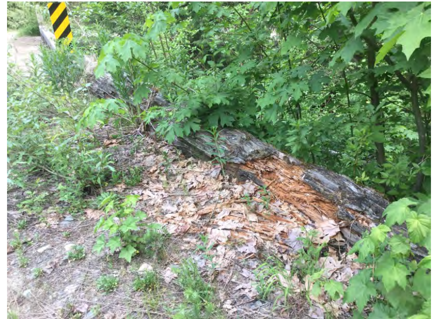
Downstream right approach fender rotten
